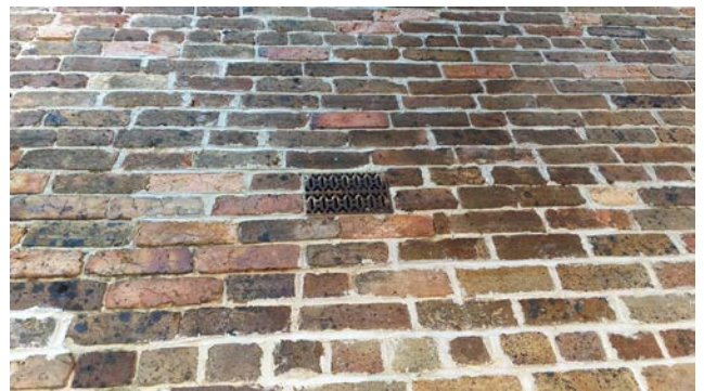
Figure 108: Metal ventilation grille and evidence of repointing on main facade facing Nimrod Street.
