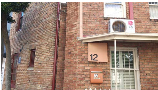
Figure 109: View of junction between the SBW Stables Theatre and neighbouring terrace house at 12 Nimrod Street. The two buildings are separated by a narrow brick wall.
